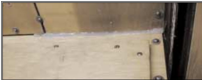
Windchest restoration goes beyond re-leathering to re-gasketing and concern for windtightness. The application of silicone sealant shown above is an expedient means of address leaks, which should have been addressed with re-gasketing.
