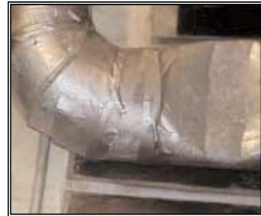
Swell duct: badly damaged, poorly repaired
