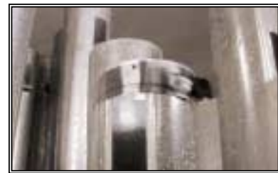
Swell pipe "repaired" with tape
