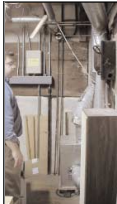
ventilation system in South chamber
