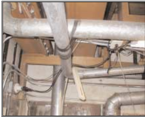
an example of sloppy 110-VAC wiring in the South chamber
