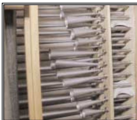
This picture does not adequately demonstrate the sub-standard method with which this vertically-mounted windchest is attached to the wall and structure. The chest moves with the slightest touch.
