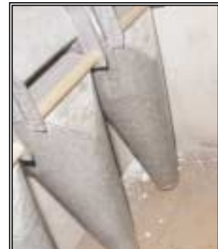
plaster dust in Choir
